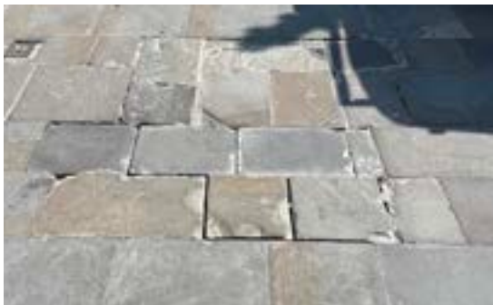
Photo 1.4.5c: Damaged paving from vehicles
