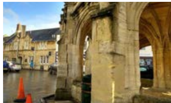
Photo 1.4.5d: Vehicle strike damage in 2018
